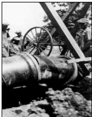
Durham City Water Works. Hillandale Plant. ca. 1920 Construction of pipeline. Workers, crane, and pipe.
